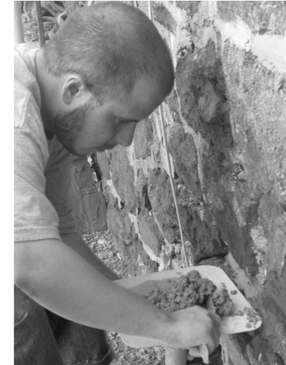
Phil is applying Lithomex, a hydraulic lime stone repair material that is used to repair damaged sections of stone. Left without repair, the damage would cause undue weathering of surrounding masonry, leading to accelerated decay of otherwise sound elements. Several different shades of Lithomex stone patch were developed because the color of the stone varied across the surface of the building.
