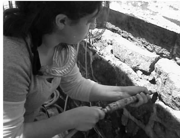
Anya uses a chisel to remove deteriorating mortar. Only mortar that was failing was removed. The goal was to save as much of the existing mortar as possible.
